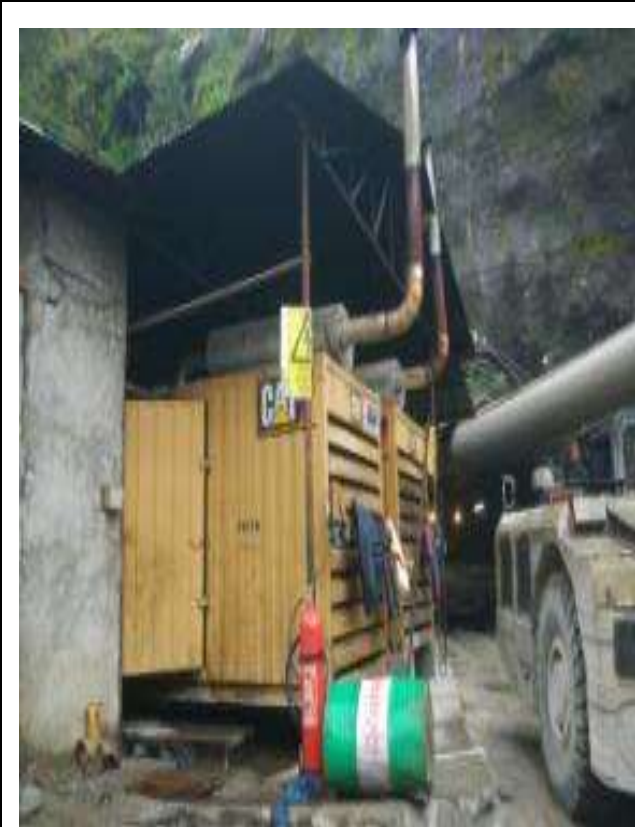
Fire extinguishers placed at DG set
